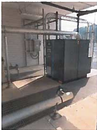
Easterly WWTF Reaeration Blower
