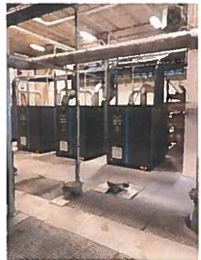
Easterly WWTF Aeration Blowers
